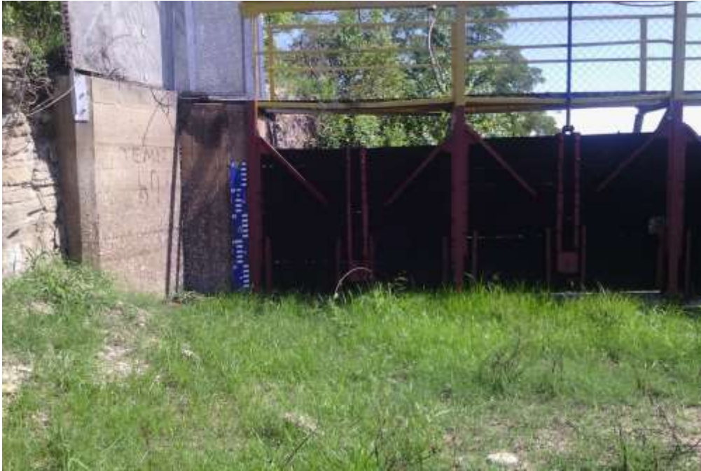
Plate 1.0: showing the low spill way gates which are still dry mid-way the rain season on the mulungushi dam.
